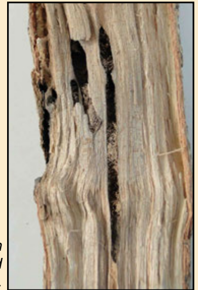
Tunnels: 1/4 inch wide and extend deep into the wood.
