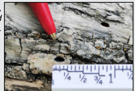
Exit holes: Oval, 3/16 inch long and half as wide.
