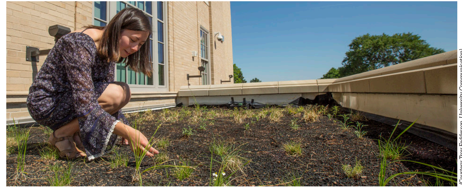
A University of Nebraska-Lincoln student looks over the grasses in a "green roof" at the university's East Campus.
